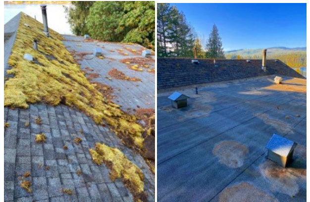
Before and after they cleaned off the roof of the main building
